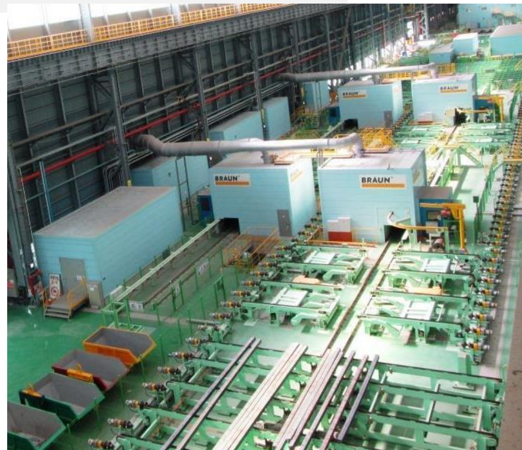
Billet grinding machines at Hyundai Steel Dangjin
