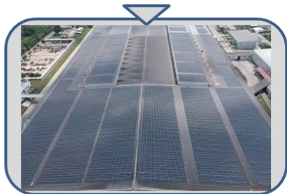
Rooftop Solar Power Plant
