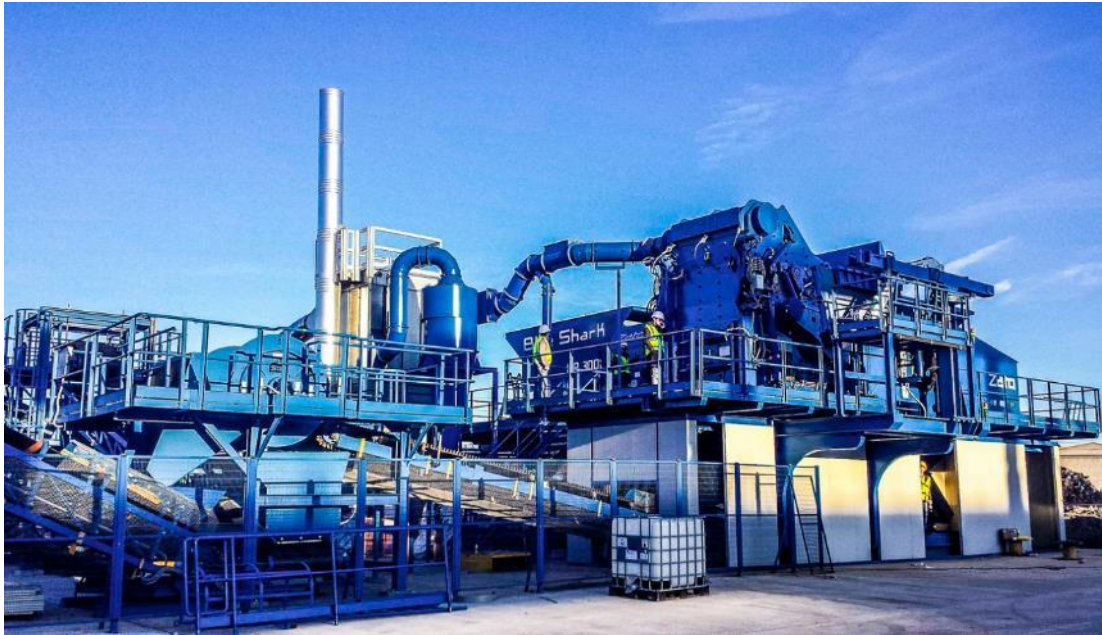
Figure 5: Hammer Mill equipped with Ferrous Recovery System – courtesy of Tata Steel UK
