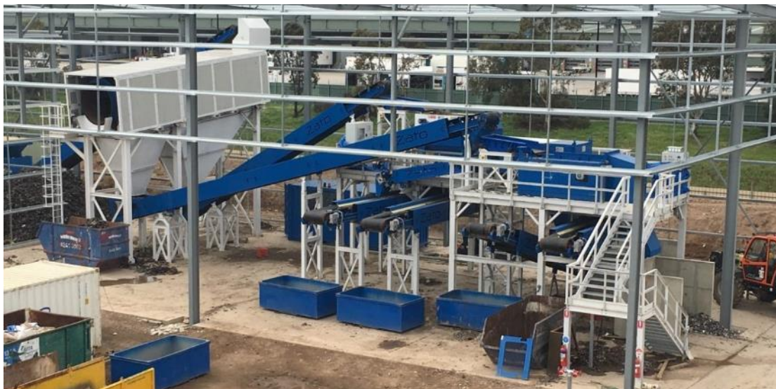
Figure 6 Downstream Plant of an Hammer Mill incl. Sieving and NonFerrous Metal Recovery – (Source Zato)
