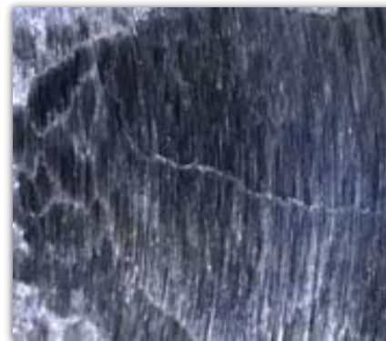
Depth of Longitudinal crack 2mm
